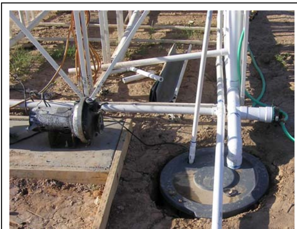
Figure 10. A underground cooling water reservoir receives the water from and delivers to glass tanks using a sump pump.
