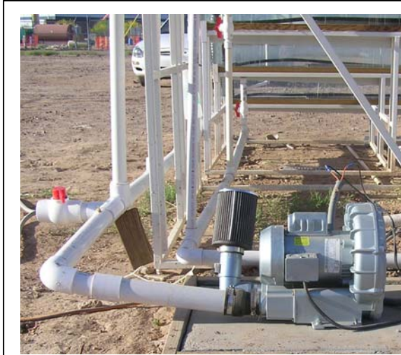
Figure 6. A Sweetwater regenerative blower for culture aeration.
