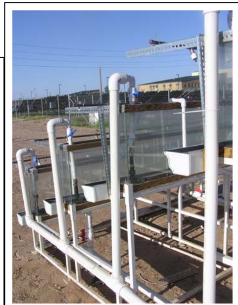
Figure 7. A PVC manifold system conveys compressed air into individual glass tanks for aeration.
