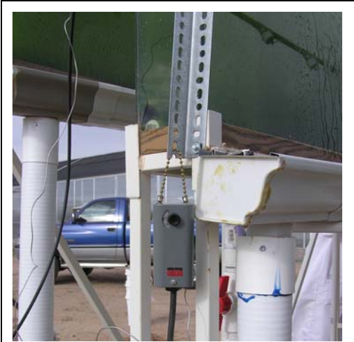
Figure 11. A thermostat installed in one tank actuates the cooling pump to delivers cooling water to misting heads for water spray when the culture temperature rises above 35°C.
